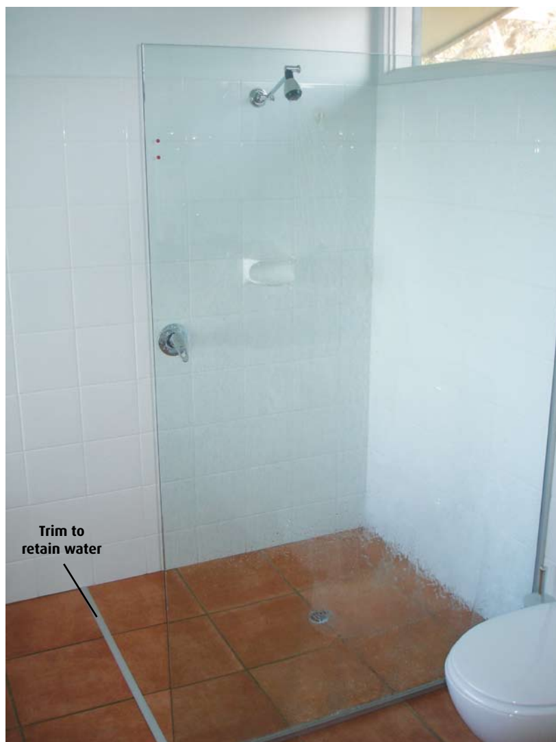
Figure 2 - typical open shower installation
